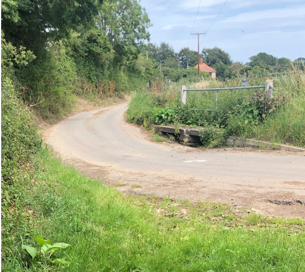
Plate 3.1: Hawthorn Road ford (photograph taken on 24.07.2020)
